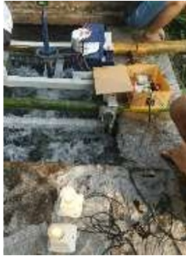
Fig 6. Experiment hydrokinetic power generation system integration in site B
