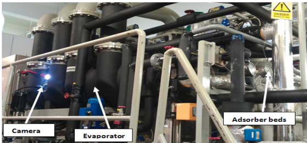
FIGURE 1. A view of AD plant showing the evaporator.
